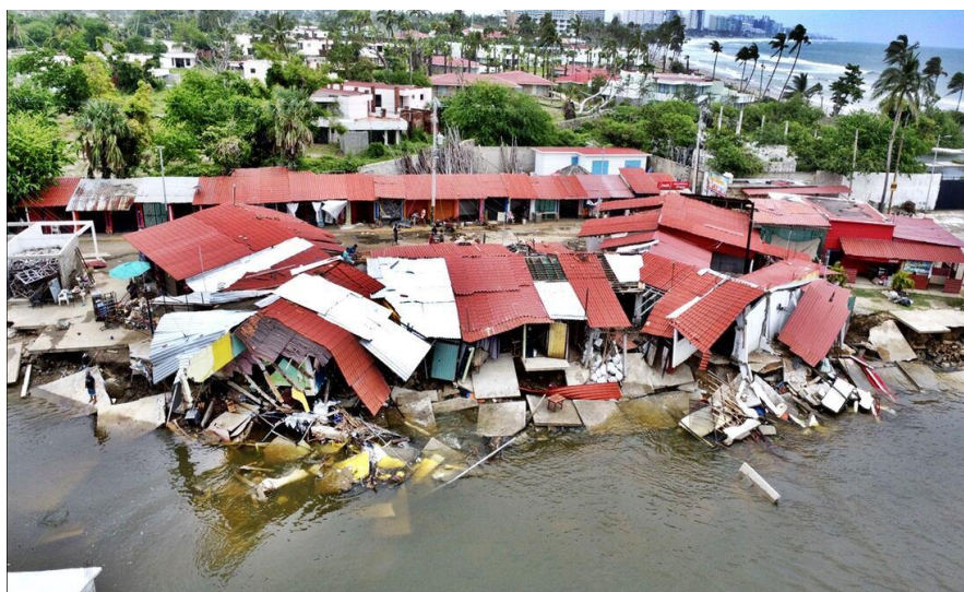
Figure 2. Flooding and destruction of roofs in Guerrero.
